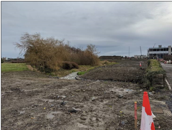
Figure 6.6 View towards realigned Baldonnel Road showing exposed sand, gravel and till (ED1) in foreground.
